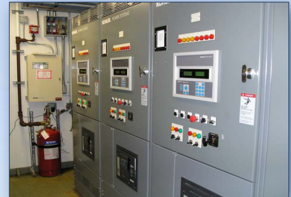
Sophisticated Kohler Power Systems control panels run some of our gen sets.
