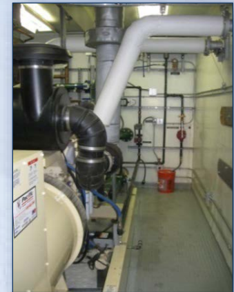
Interior of a generator module.
