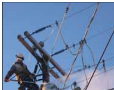
Sam Lindquist powerwashed Savoonga's storm-damaged facilities.
