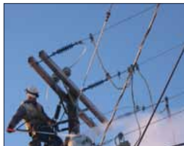
Sam Lindquist powerwashed Savoonga's storm-damaged facilities.
