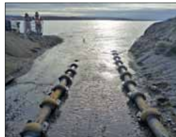
The ends of the Brevig Mission-Teller submarine cables are covered by protective armor.
