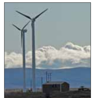
Shaktoolik's two wind turbines.
