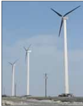
Three of the four wind turbines in Emmonak.
