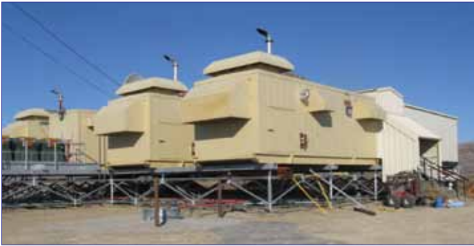
The new Brevig Mission power plant sits on a tridetic foundation.
