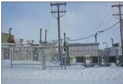
Emmonak's old power plant, first built in 1970.
