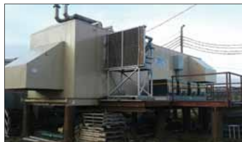
Alakanuk's new stand-by power module.
